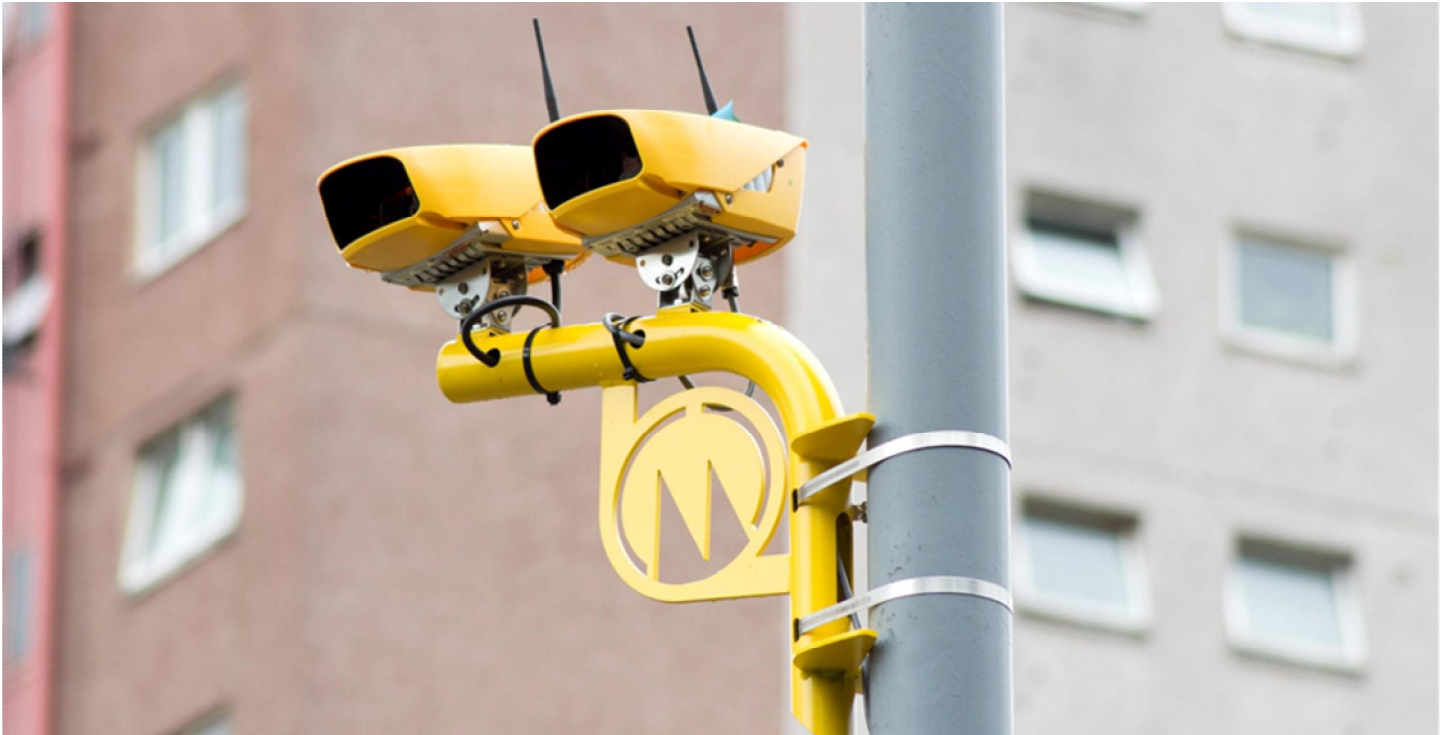
Low cost, spot speed replacement SPECS installation using highly distinctive street lighting brackets (West Midlands).
